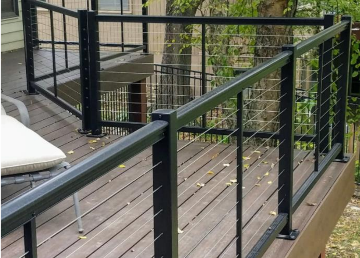
GUARDRAIL – STAINLESS STEEL CABLE IRON RAILING
