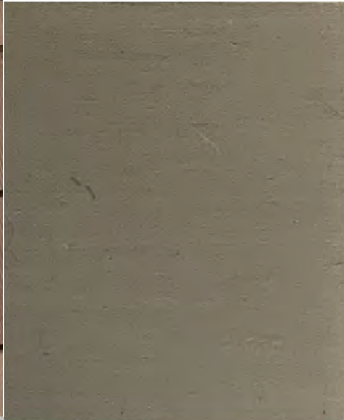
STANDING SEAM ROOFING TERN METAL
